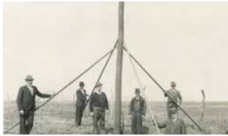
First Access Energy Cooperative pole being set at the Parke F. Cornick residence.
