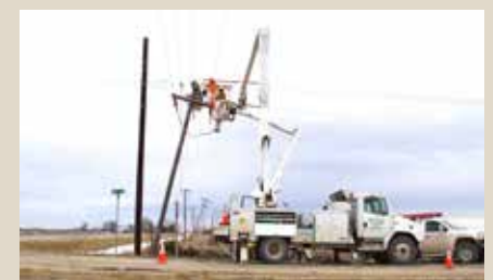
Cost to install a pole today over $2000
